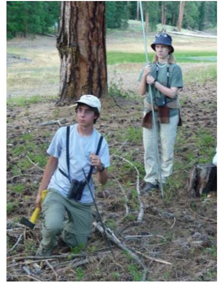
Eric and Marissa place rebar and poles at a net site near Lake McDaniel
